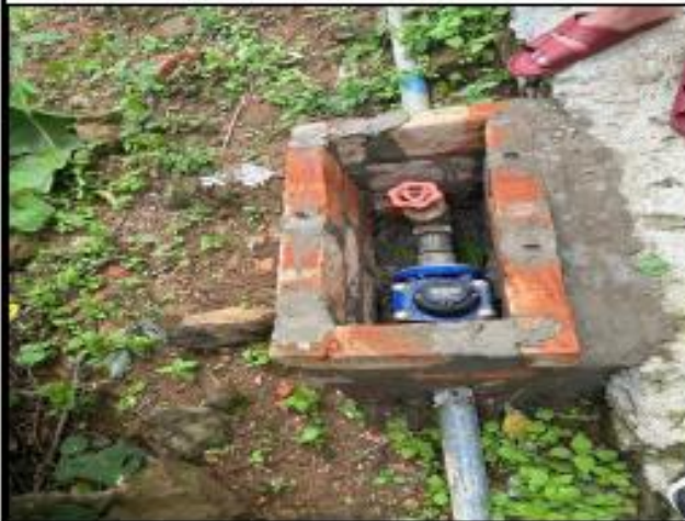
Photo : Gravity main line
